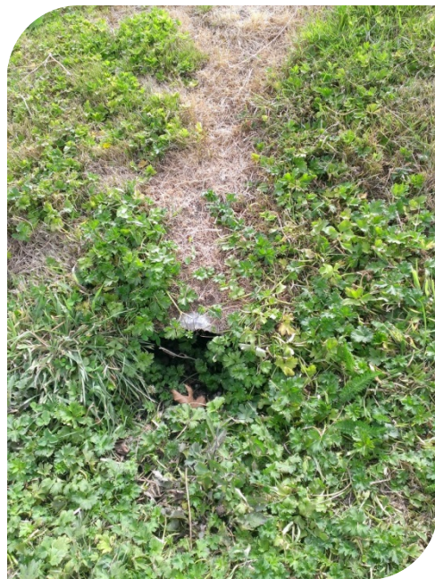
Photo 10— Outlet downslope of catch basin. Note lack of channel.
